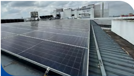
All our owned-rooftops are now equipped with solar PV systems.
